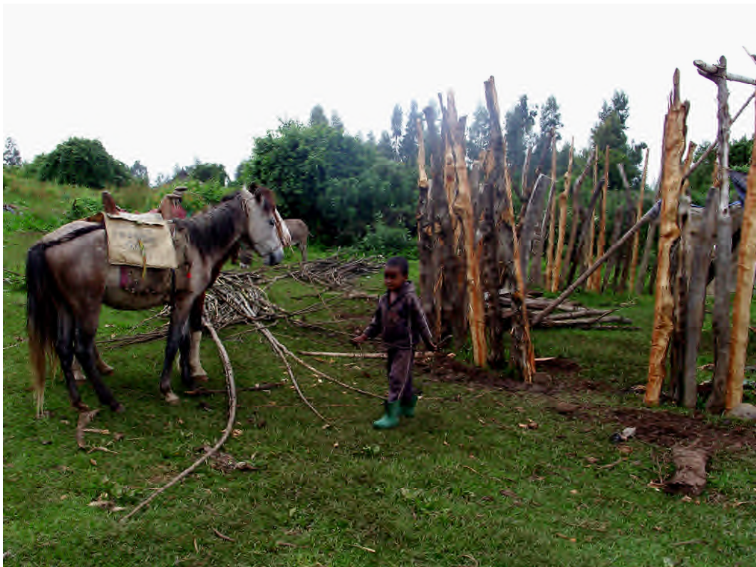
Plate 4.5: A new house in the process of being constructed, with the frame made from J. procera wood.
